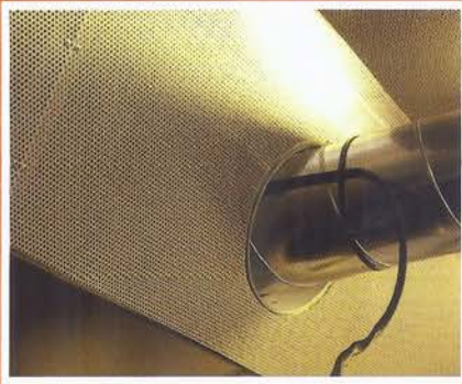
Sound Proofed Container Insulation Stainless Steel Coverage.
