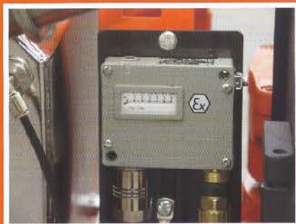
Ex Shut down pressure switch.
